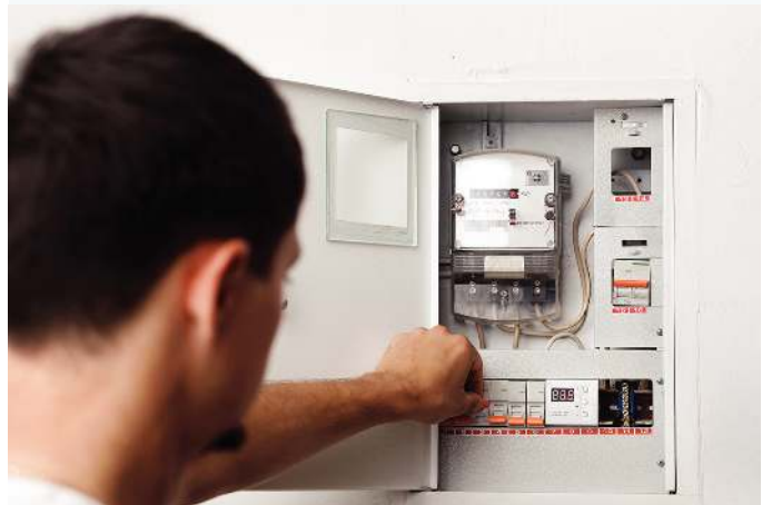
FIGURE 5.3 Many houses have a meter and circuit breaker in their meter box. The circuit breaker is in the bottom left corner.
