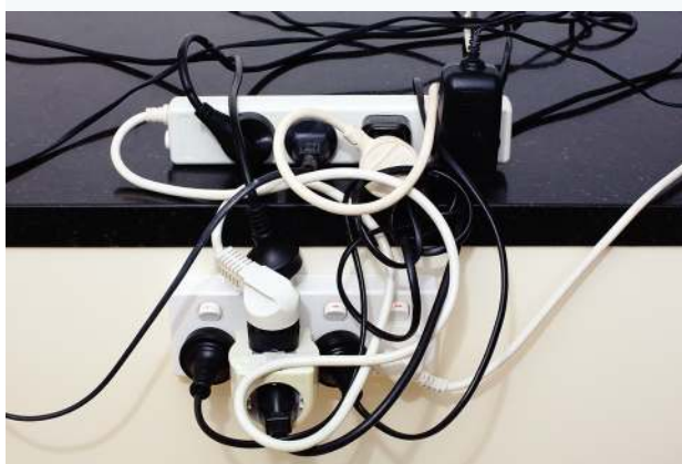
FIGURE 5.12 Overloading of an electric circuit
