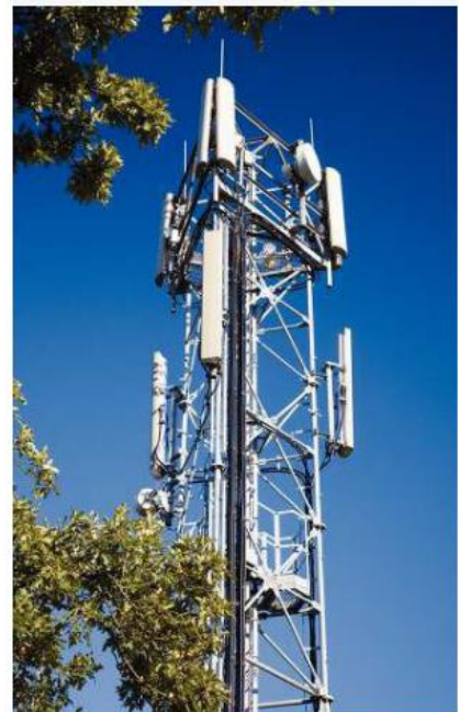
FIGURE 8.12 Hundreds of mobile phone towers around the state receive and transmit radio waves from mobile phones.
