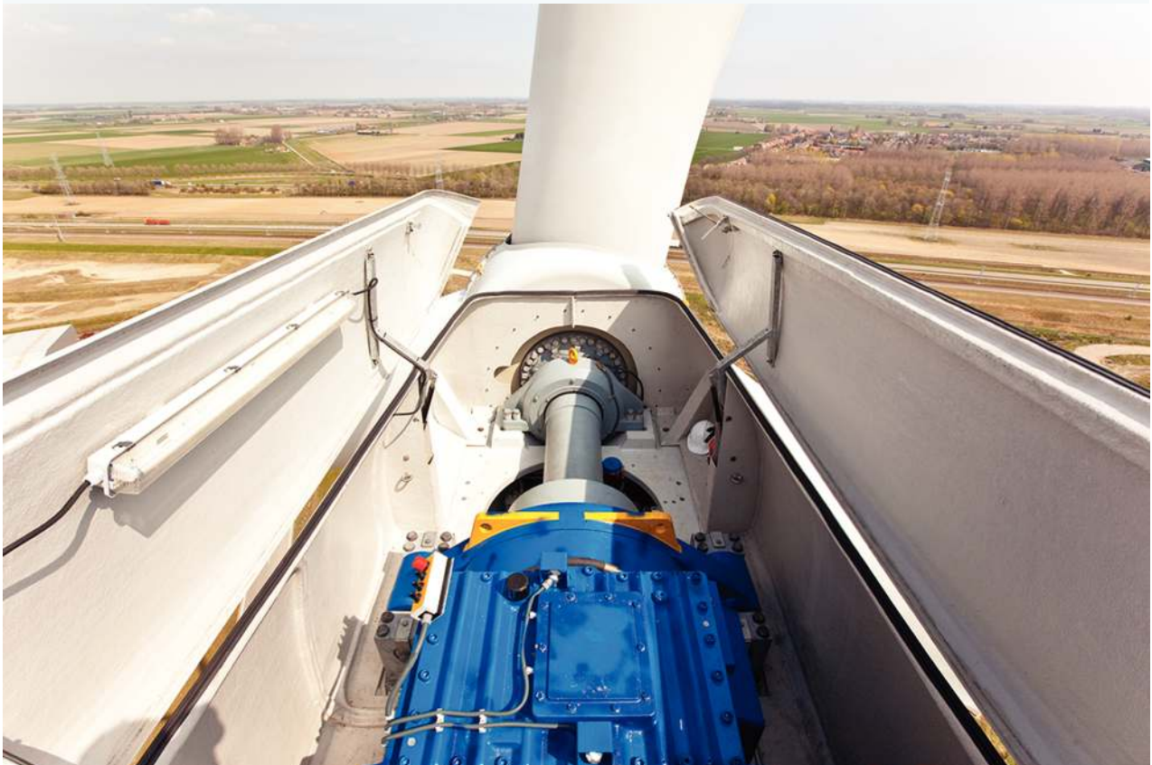
FIGURE 4.1 A generator inside a wind turbine
