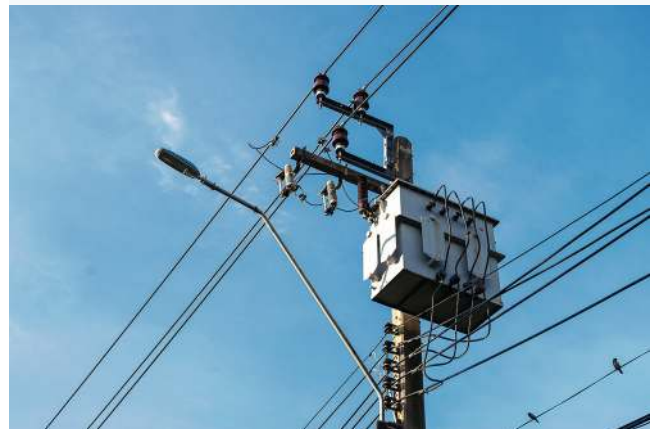
FIGURE 5.9 A pole transformer
