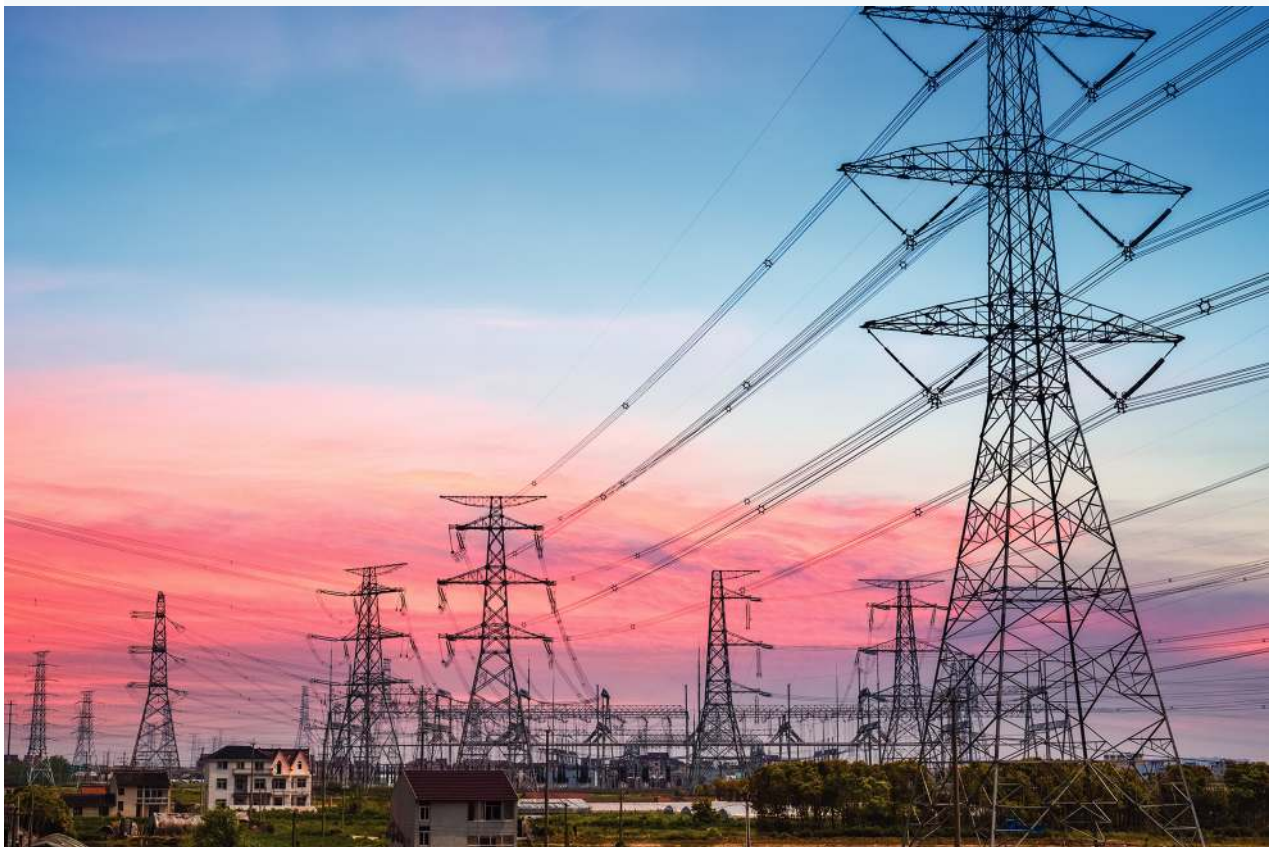
FIGURE 5.1 High-voltage power lines are used to transmit electricity over long distances.
