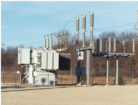
FIGURE 5.8 A transformer at a substation
