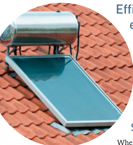
Figure 3.59 Solar panels can be used to heat water for your house.
