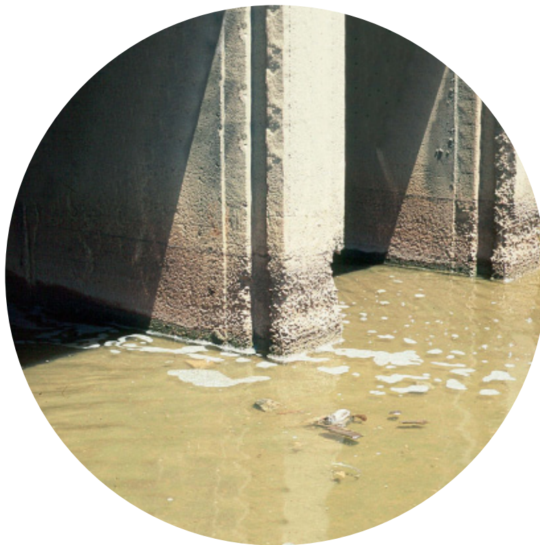
Figure 5.65 This concrete bridge pylon is being destroyed by sulfuric acid from acid sulfate soils, which reacts with the carbonate in the concrete.
