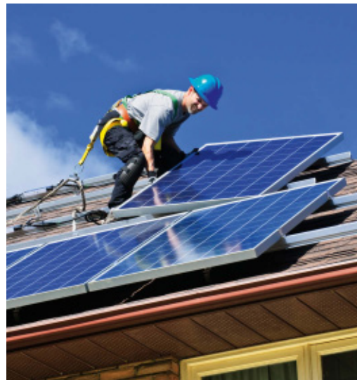
Figure 3.60 Installing solar panels on your roof could make a big difference to your electricity bills. It is something your household should consider?
