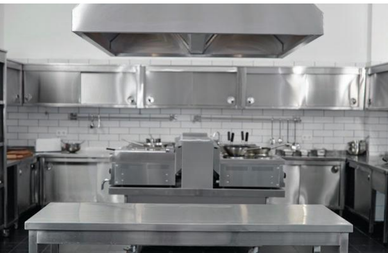
Figure 12.35 Ensure all equipment is clean and well maintained.
