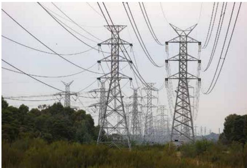
Transmission lines and towers near Melbourne
