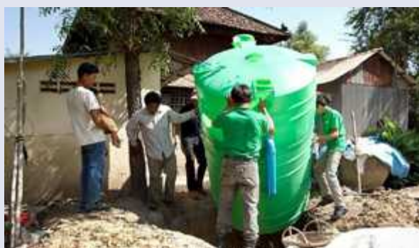
Figure 3.02: Bio-digesters are finding success in countries such as Cambodia.
