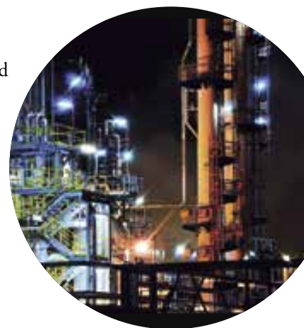
Figure 4.6 In oil refineries, distillation towers are used to isolate the different liquid fractions in crude oil.
