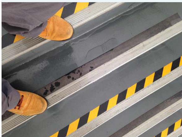
FIGURE 3 Reference image 2 taken at 3.18 pm on 21 May 2021, Low-Water Public Swimming Pool, exit stairs by the north gate, loose and missing warning tapes
