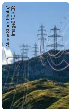
▲ FIGURE 5.5.1 The properties of aluminium make it well-suited to span long distances between power poles.
