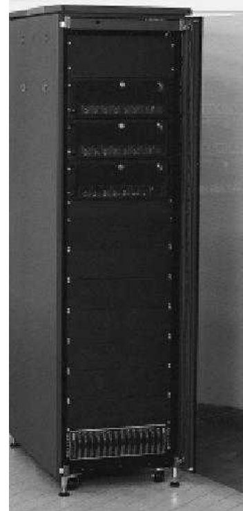
Fig 2.24 This server has some 3000 gigabytes of storage and is able to transmit up to 2500 megabits per second.
